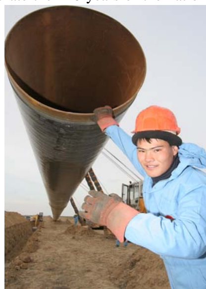
Pipe dreams come true... A Kazakh worker helps lay a pipe for a new export oil pipeline.
